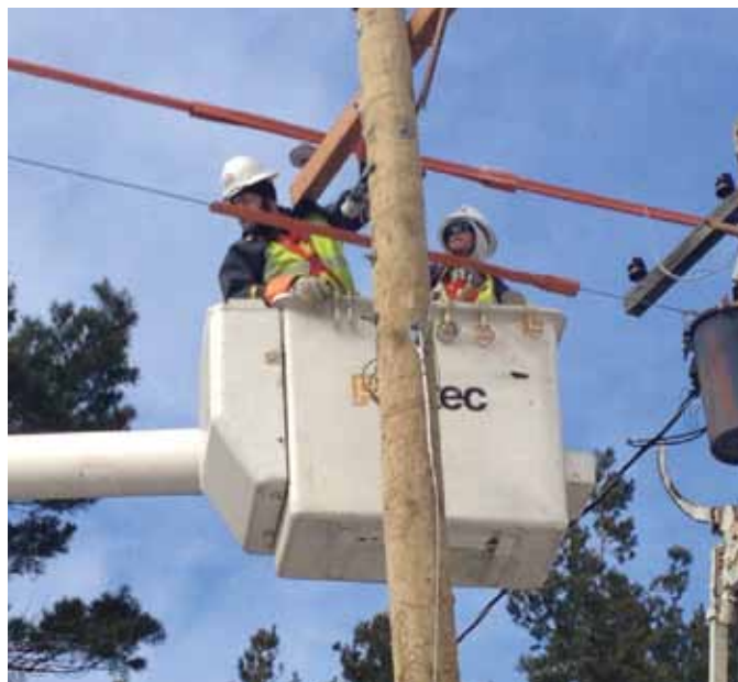
Lineworkers Jeremy Zbytowski and Kyle Balderson are shown connecting a newly-installed utility pole to the system (the old pole and transformer are shown at right.) Crew leader Chris Teachout directs from the ground.
