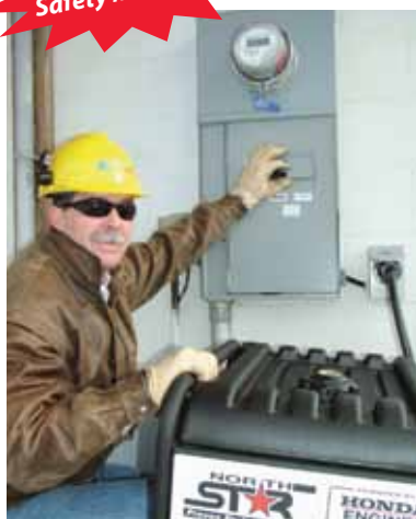
Dave Matz, Great Lakes Energy’s operations director, points out the safety transfer switch that allows a portable generator to be safely connected to a home.
