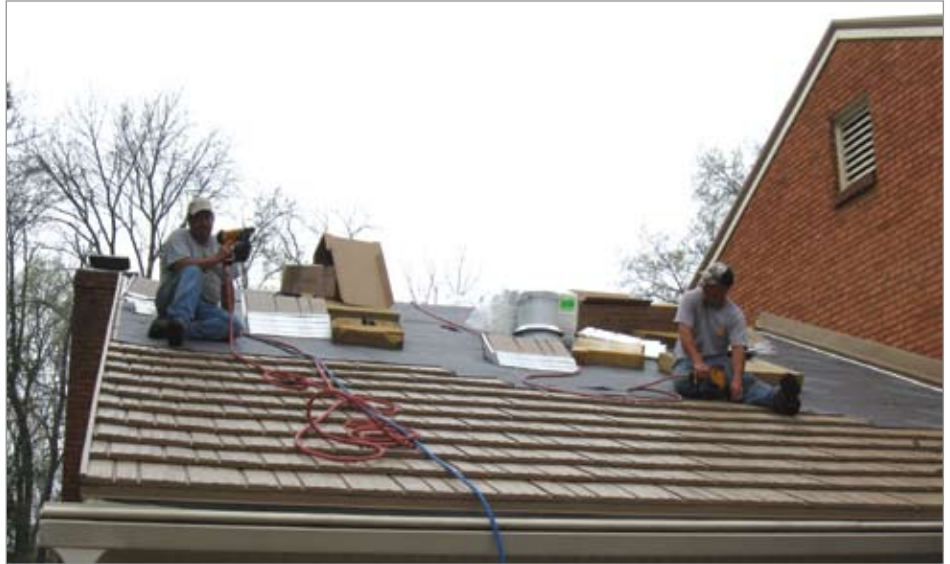
The metal roofing panels are installed over the underlayment. Hidden stainless steel nails and aluminum clips are used to secure each panel.
