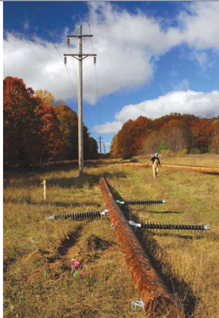
Transmission system improvements, such as this pole replacement project in Mecosta County, help Wolverine Power Cooperative deliver reliable power to Great Lakes Energy and other members who rely on Wolverine for their power supply.
