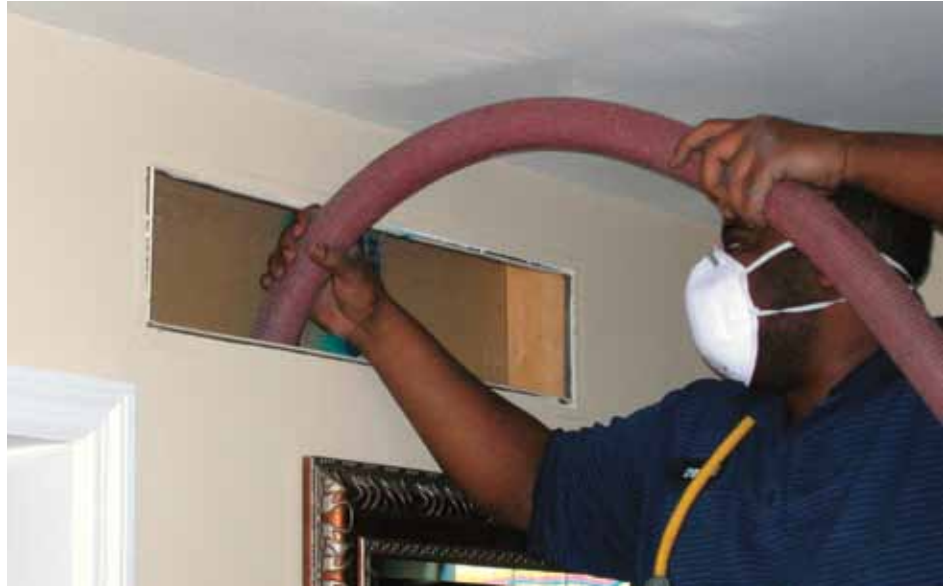
A long vacuum hose is inserted into the wall return duct. It is connected to an indoor vacuum unit with a HEPA exhaust filter.
