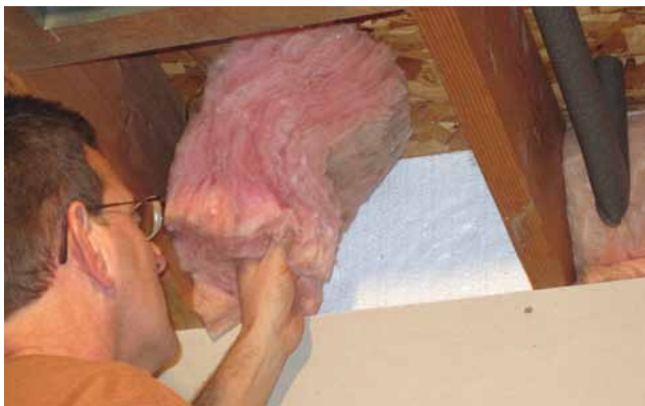
Kevin Cragg replaces insulation batting after inserting a 2-inch-thick piece of foam board insulation (R-7.8). Spray foam insulation was used to seal around the foam board, as needed. ►
