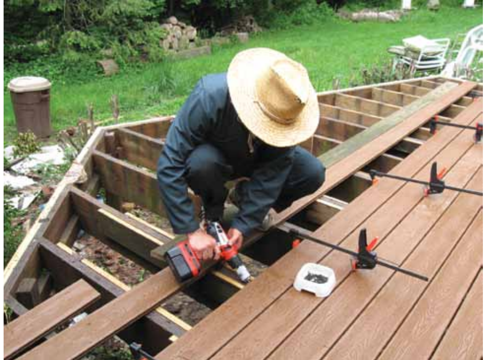
James Dulley is shown installing composite decking using hidden fasteners. Since these planks are not as rigid as wood, it is important to make sure you have proper maximum spacing between the joists.
