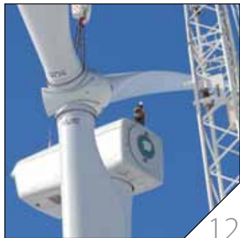
Photo - Basin Electric
