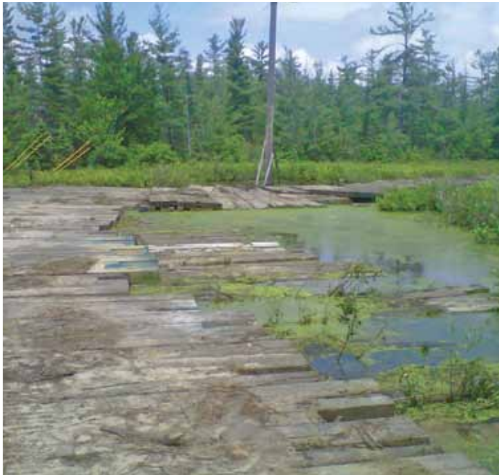
Rebuilding a transmission line near Shelby took extra effort this summer. A special pole measuring 110 feet and set 28 feet deep was needed to reconstruct a line segment located in a wetland area. The typical transmission pole is 85 feet. Lineworkers laid a track for equipment needed to complete the task.
