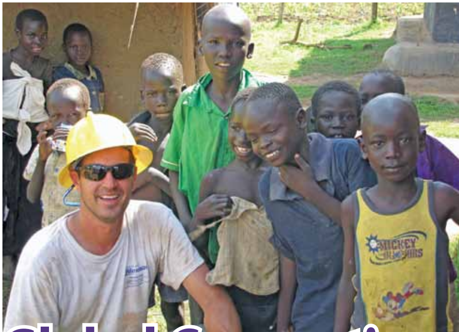
Volunteer lineman Phil Hogan from Habersham EMC in Georgia takes a break from wiring new utility poles to spend time with local children in Yei, Sudan.
