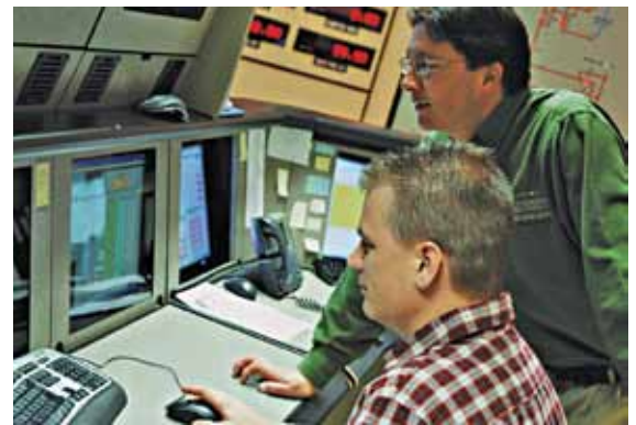
Justin Russell (foreground) and Mike Anderson monitor power supply in Wolverine’s Energy Control Center.
