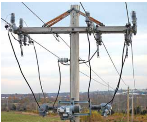
Reclosers protect lines and consumers from short circuits and allow temporary faults to clear, which helps keep service energized without needless interruptions.
