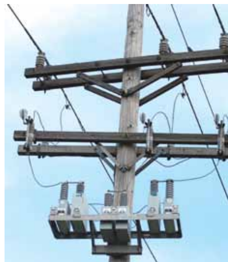
Capacitors improve the power on the lines—they prevent it from being wasted and help boost the voltage on long distribution lines.
