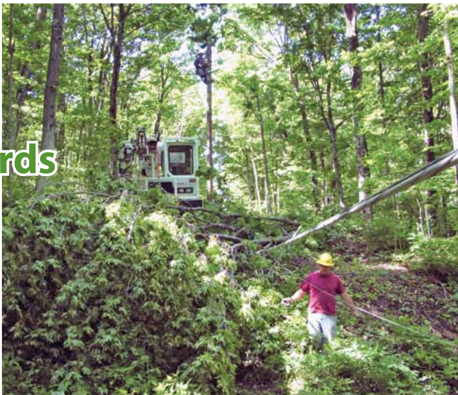
Great Lakes Energy crews rebuild a power line knocked down by trees during a summer storm last year.
