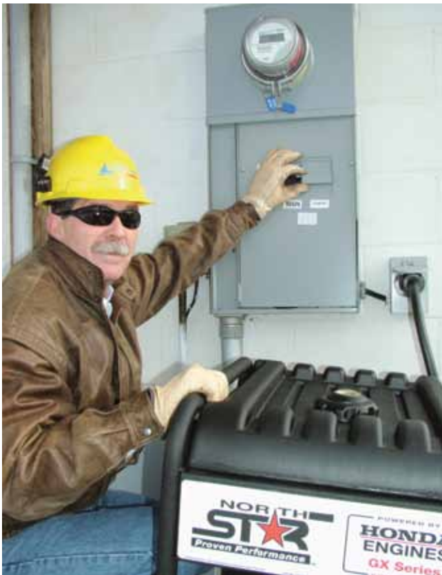
Dave Matz, Great Lakes Energy's operations director, points out the safety transfer switch that allows a portable generator to be safely connected to a home.
