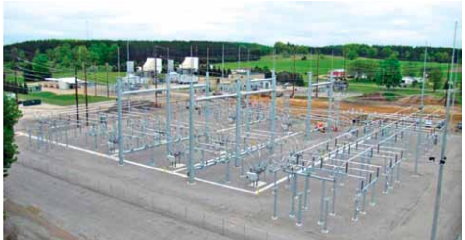
Wolverine's new Hersey transmission substation, completed in April 2011.
