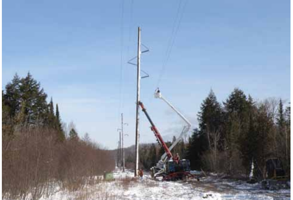
Wolverine lineworkers upgraded a section of the transmission system between Petoskey and Boyne City in February 2011 by installing new poles and wire.
