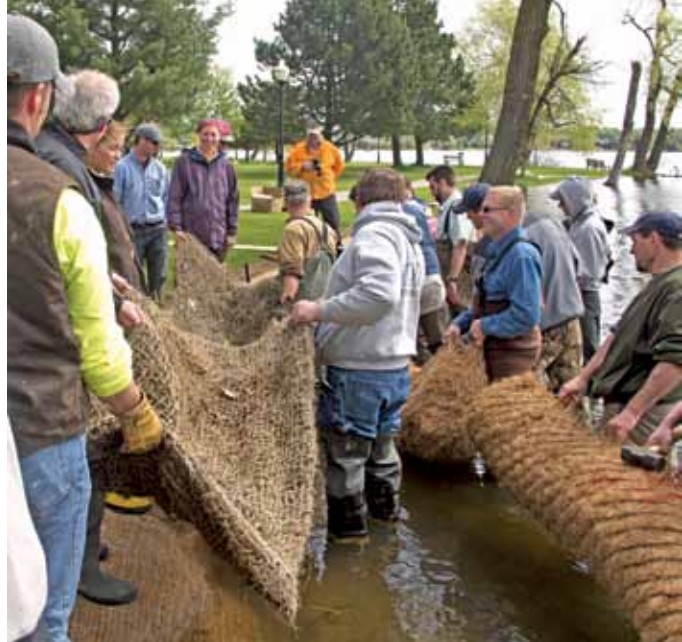
During the field component of training for becoming a Certified National Shoreline Professional, participants lay erosion control fabric and set coir fiber logs as wave breaks to protect the newly-constructed natural shoreline at Cadillac Lakefront Park.
