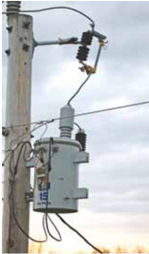
Transformers lower voltage to a level that's safe for use in your home.
