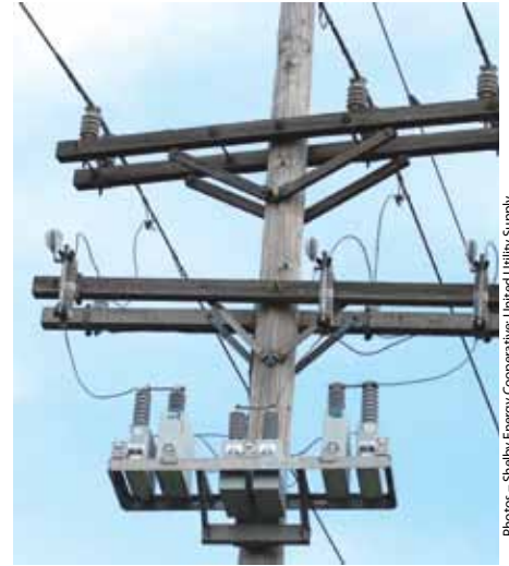
Capacitors improve the power on the lines—they prevent it from being wasted and help boost the voltage on long distribution lines.
