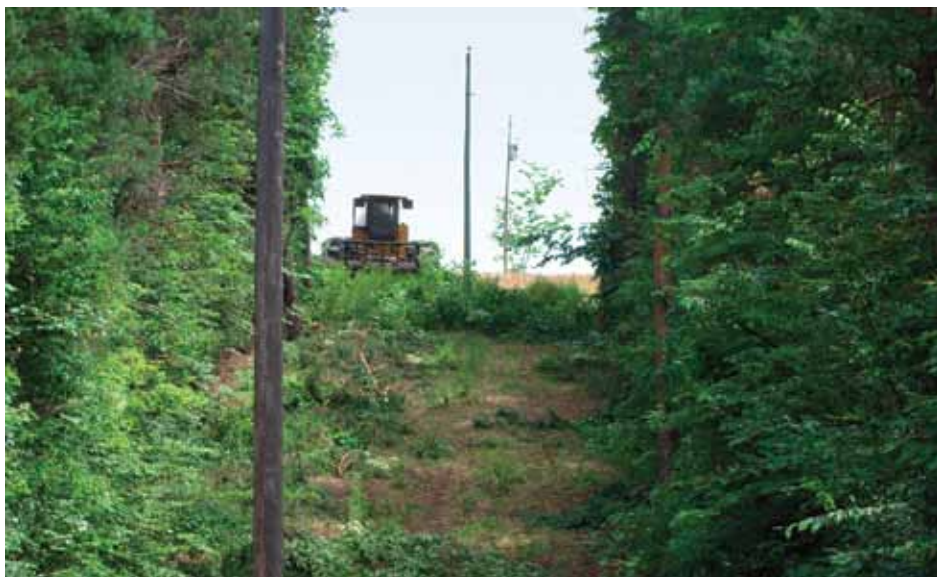
Private contractor crews will work in 2012 to remove trees near power lines for safer and more reliable electric service for Great Lakes Energy members.
