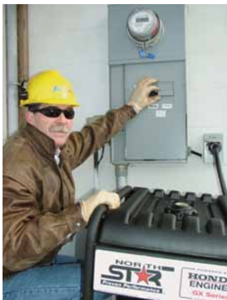
Great Lakes Energy's Dave Matz holds the utility/generator transfer switch that protects lineworkers and the home when a portable generator is in use.
