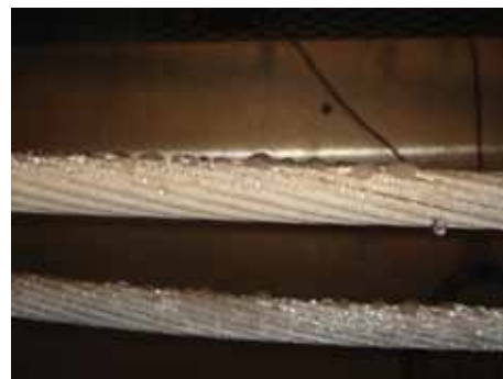
Lines treated with a superhydrophobic coating repel liquids and prevent major ice accumulation. Any ice that might sit on the lines would be easily blown off by wind or vibration from the power flow.
