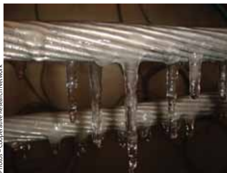
When freezing rain accumulates on electric lines, they become extremely heavy, often breaking and toppling support poles, which leads to power outages.
