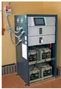
Home battery backup units (shown without a cover) are about the size of a refrigerator and generally fit in basements or spare rooms.
