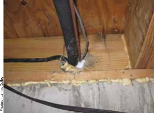
Check for gaps and air leaks where the sill plate rests on the top of the foundation.
