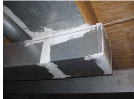
Seal seams in the ductwork where there are visible gaps or you can feel heated or cooled air leakage.
