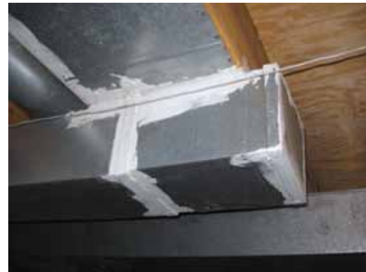
Seal seams in the ductwork where there are visible gaps or you can feel heated or cooled air leakage.
