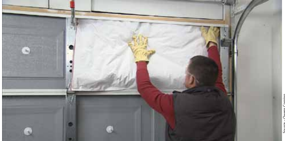
After clips are stuck to the garage door, fiberglass insulation batts are pressed over the clips.
