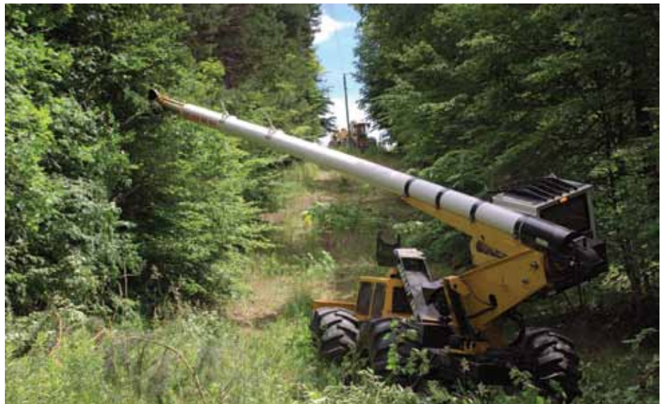
Private contractor crews will work in 2013 to remove trees near power lines for safer and more reliable electric service for Great Lakes Energy members.
