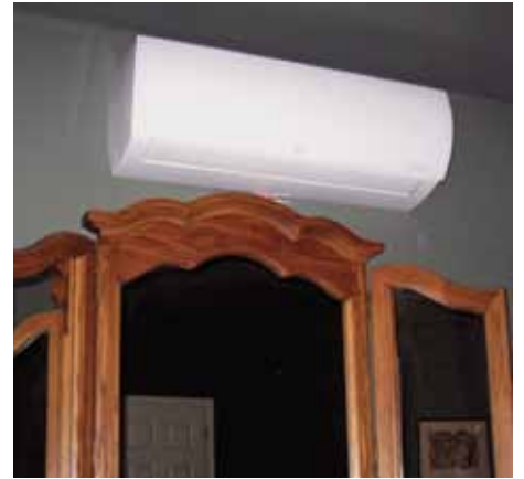
The indoor fan/coil unit is mounted high on the bedroom wall.
