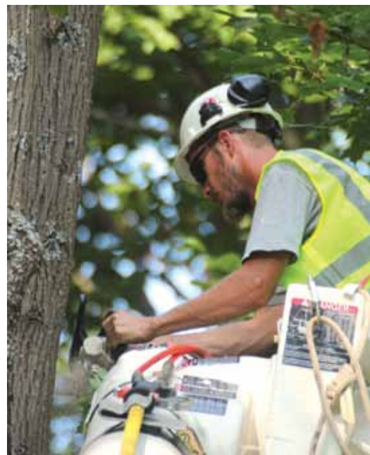
A contracted worker removes a tree near Great Lakes Energy power lines. It is one of 3,400 dead, dying and diseased trees removed so far since a new vegetation management program to reduce tree-related outages was started last year.
