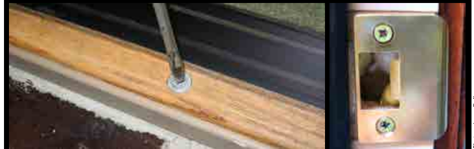
LEFT: A door's threshold can be raised or lowered with a screwdriver so the weather stripping seals tightly. RIGHT: Stepped teeth in this strike plate allow the door to fit tightly. Notice the small dab of expandable foam insulation inside.
