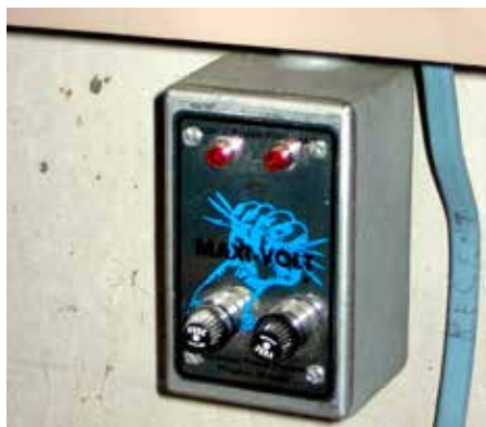
A surge protection device can be mounted at the base of your main electrical panel.
