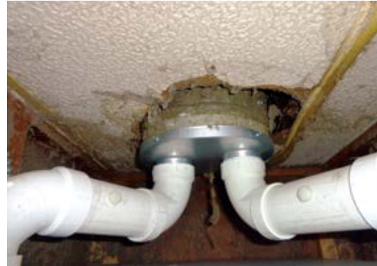
Fig. 1—A large chimney hole is a huge energy loser. It can be sealed with sheetrock, then caulked air-tight.
