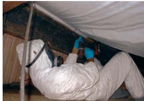
Fig. 2—Underneath the home, a "sling-patch" can be screwed into the inner side of the I-beam. It stretches to the other I-beam and holds insulation under the ductwork in place.
