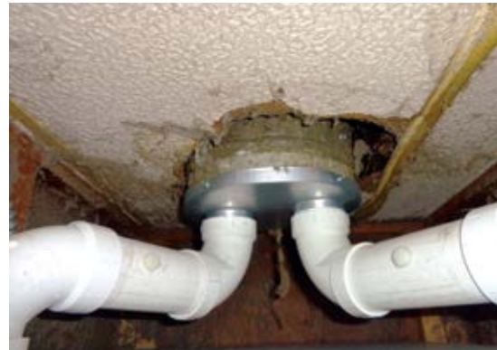
Fig. 1—A large chimney hole is a huge energy loser. It can be sealed with sheetrock, then caulked air-tight.
