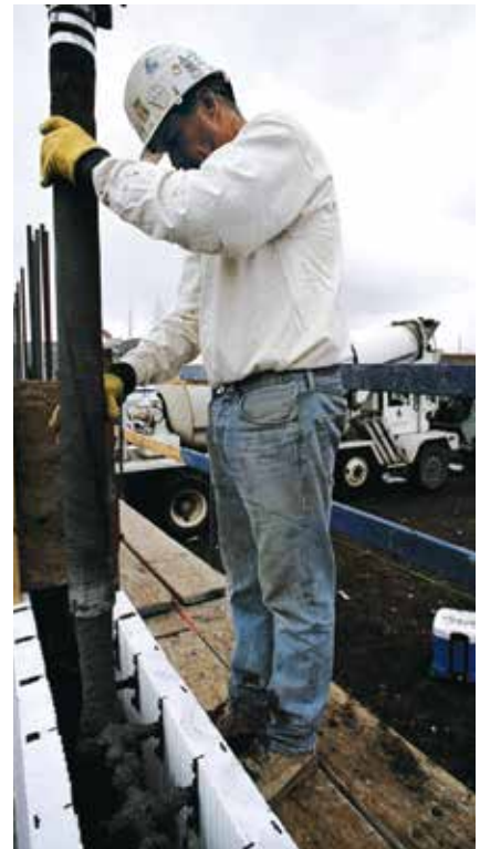
With “stay-in-place” construction, once the insulated forms are erected and reinforced steel installed, the concrete is pumped in from the top.
