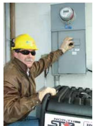
Great Lakes Energy's Dave Matz flips the transfer switch on the meter base for safely operating a portable generator.
