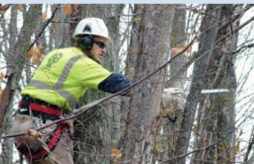
Contracted tree-trimming crews are again working this year to remove trees that pose a threat to power lines.
