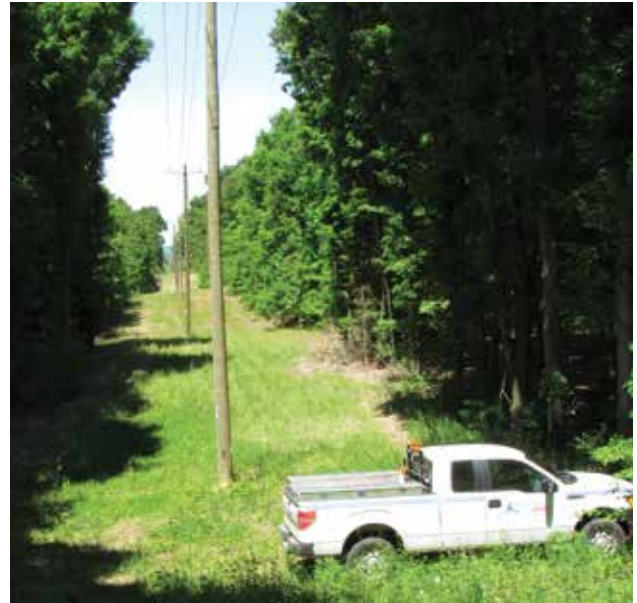
Great Lakes Energy uses the right-of-way to build and maintain its power lines and to manage trees and other vegetation within it that could pose a threat to your electric service.
