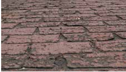
Failed asphalt shingles cracking and peeling.
